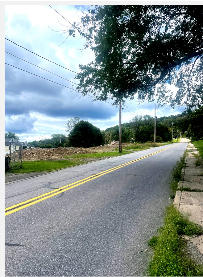
Northern view of the corridor, featuring the demolition site of the old Penneco homes.
